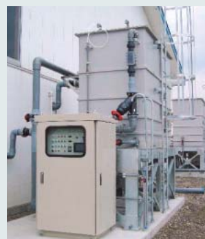
Water treatment equipment
